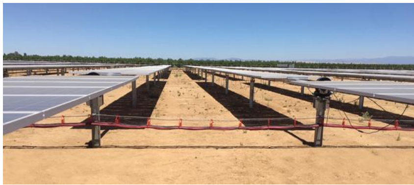
Shown: CAB/BLA Above-ground DC Cables
